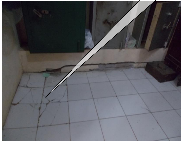
Deflection at 1st floor, Indication of foundation settlement
